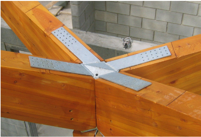
Figure 3. Detail of single shear rivet connection on 4 different members. The weldment was detailed so that each glulam members would be slid in place. The rivets need to be installed next.
