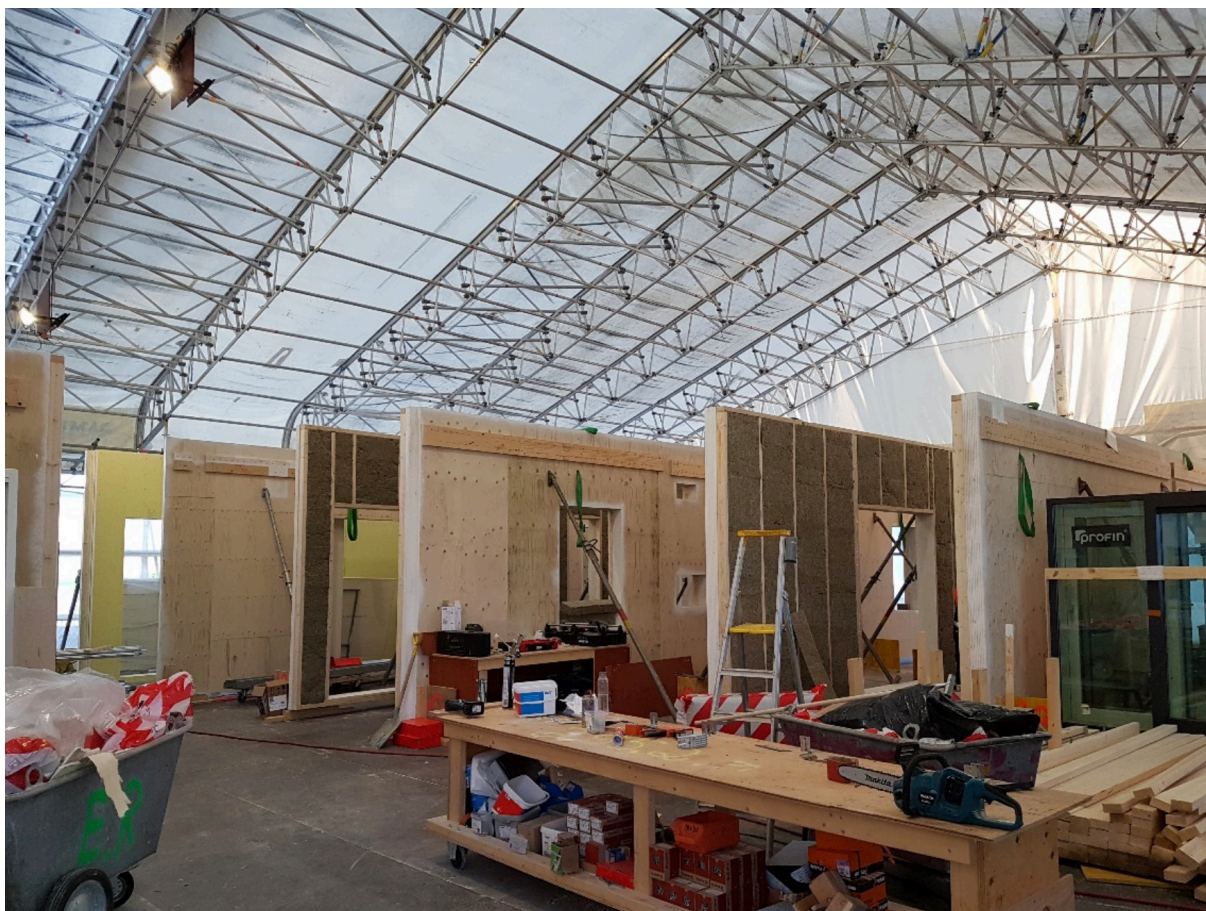
Figure 9: Picture taken from inside of the prefabrication tent located next to building site. Courtesy of Rakennustoimisto Reijonen.
